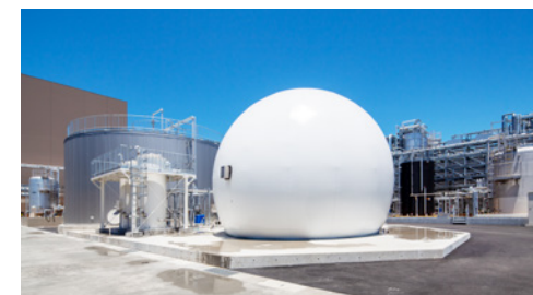
Methane fermentation plant at the Setouchi Hiroshima Factory
