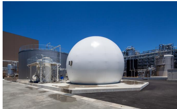
Methane fermentation tank, desulfurization equipment, gas holder, etc.
